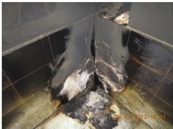
Figure 3: Scene of incident (Bath room).
